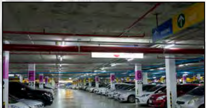
Car Park Ventilation
